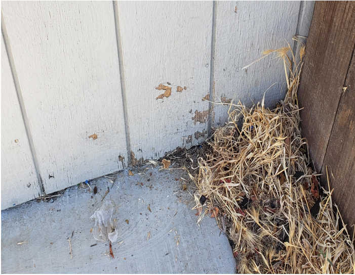
2A - DRYWOOD TERMITE
